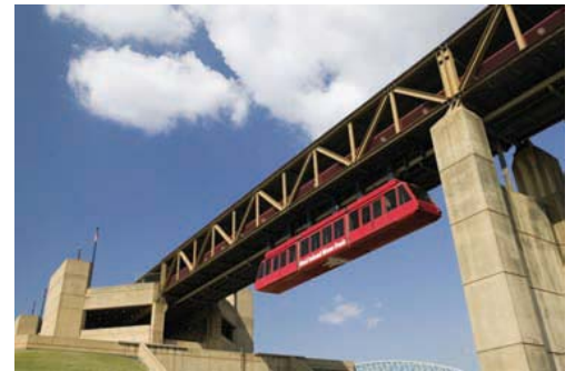
Photo 1.2 This bridge truss consists of two-force members that may be in tension or in compression.
